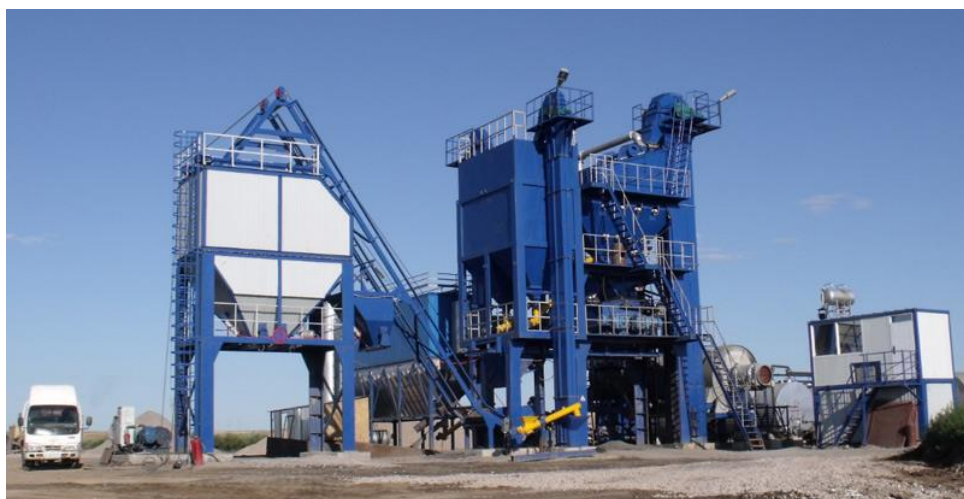
Gambar 3. 11 Asphalt Mixing Plant (AMP)
